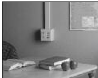
2400 Series Raceway shown with our new 2444D-2N Divided Device Box in a typical classroom application.
